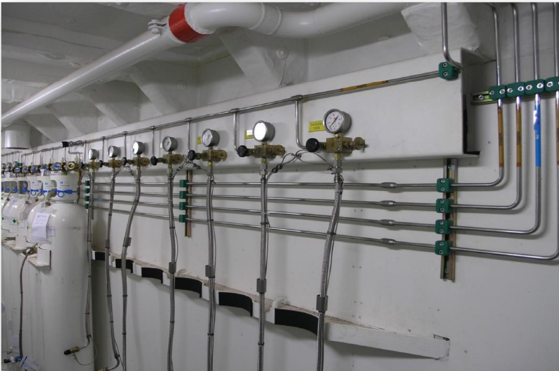
Example of an oxygen distribution installation
